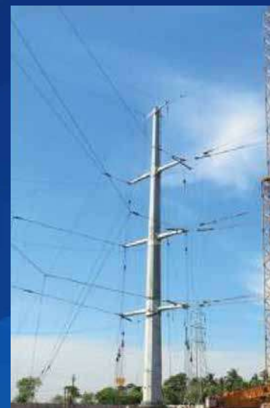
400kV D/C Quad Moose Monopole
