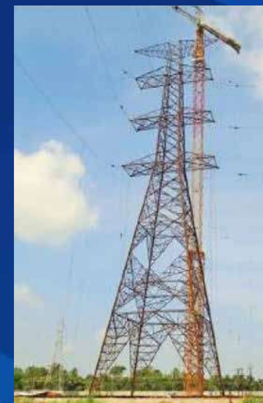
500kV Transmission Tower
