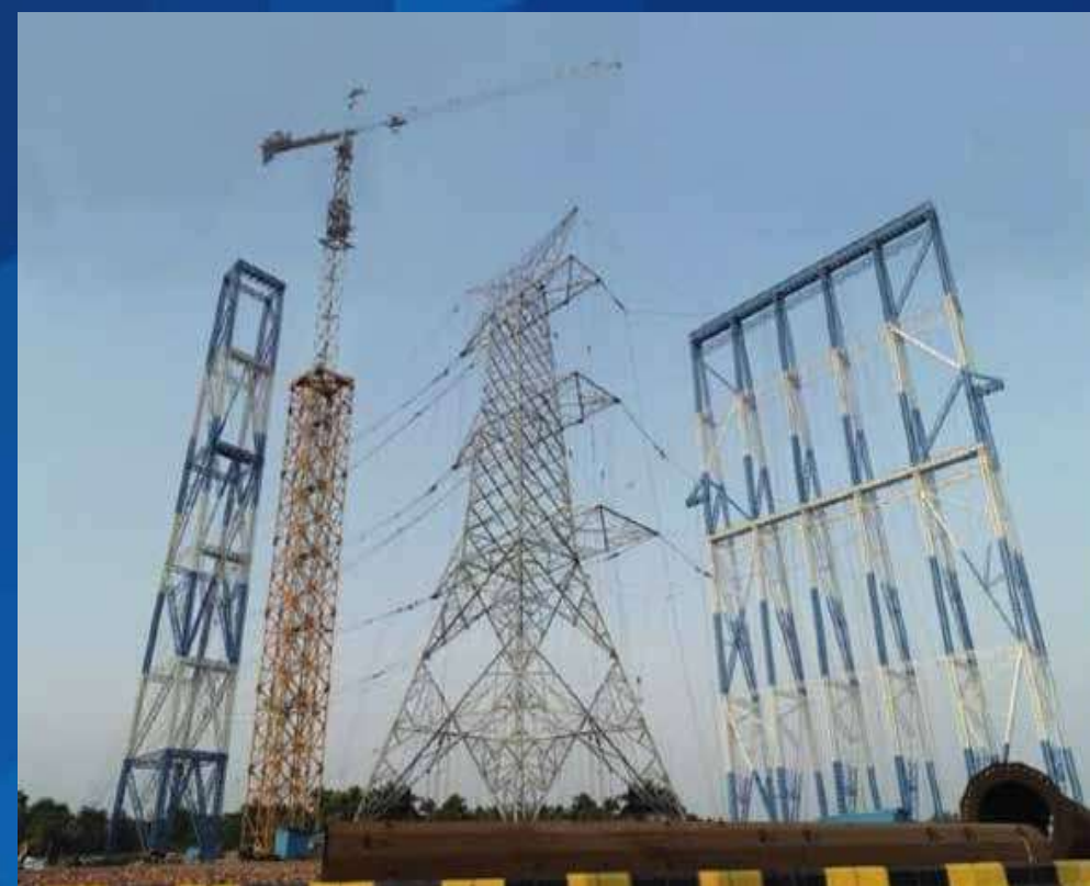
765kV Transmission Tower
