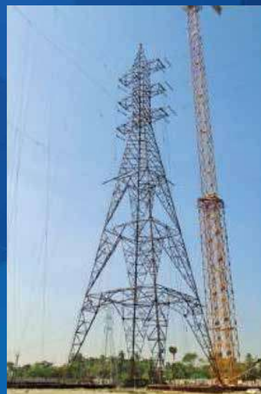
220kV Transmission Tower
