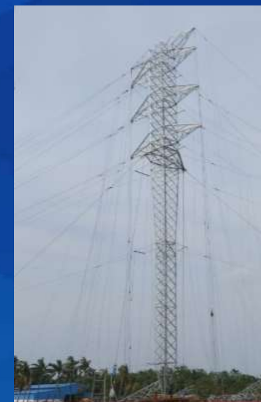
300kV Guyed Transmission Tower
